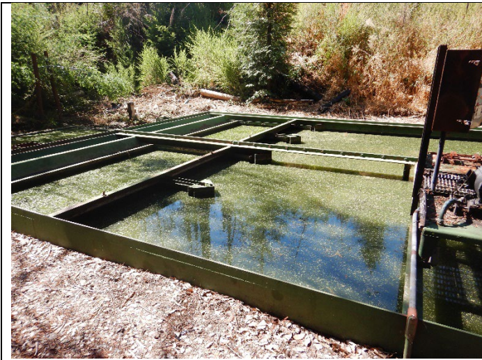
Figure 3. Activated sludge basin acting as a holding basin for untreated domestic wastewater
