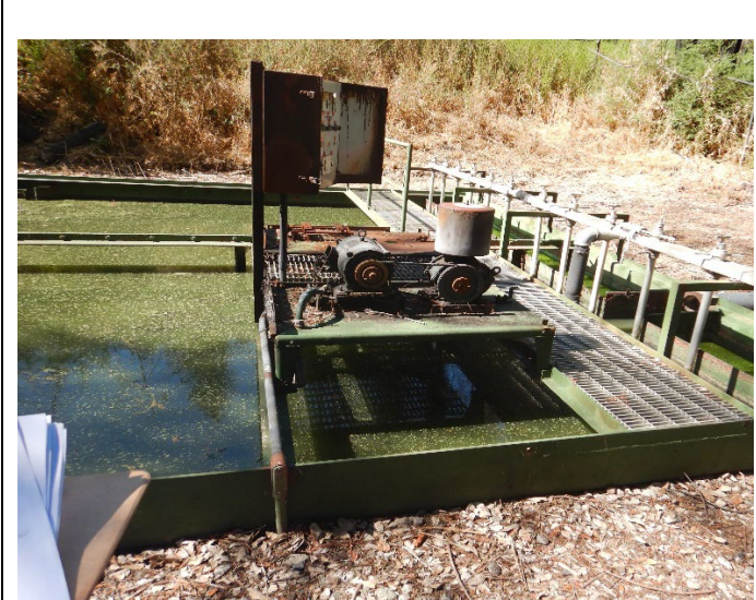
Figure 5. Existing Aerator motor impacted by fire damage
