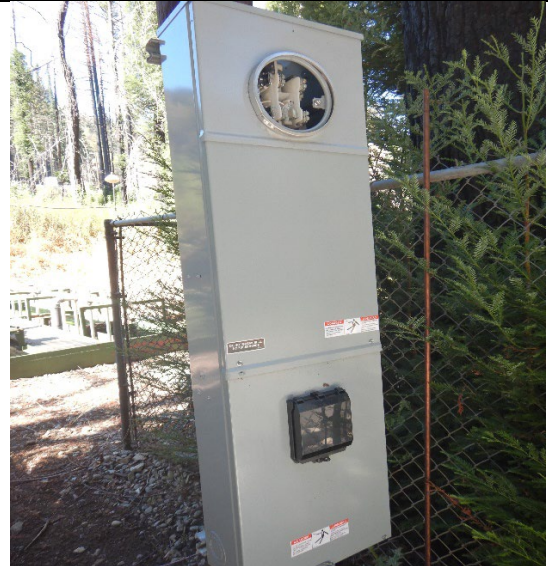
Figure 8. New incomplete electrical box
