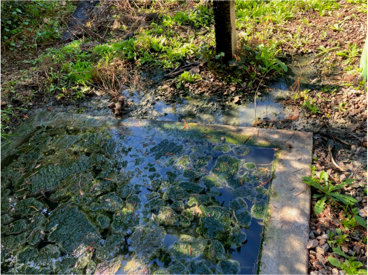
Figure 7: Untreated wastewater overflowing basin Photo provided by Nader Sidhom, Vector Control Specialist, Santa Cruz County Mosquito and Vector Control and taken on October 27, 2022
