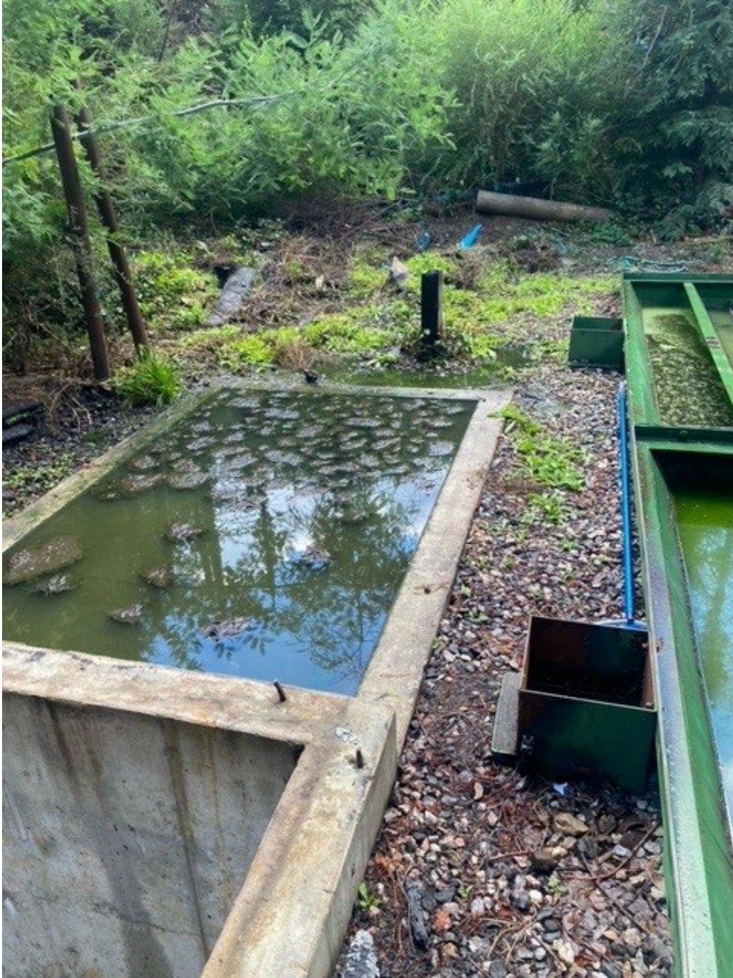
Figure 6: Untreated wastewater overflowing basin Photo taken by Kristy Emershy, California Department of Fish and Wildlife, Santa Cruz Harbor District on November 2, 2022
