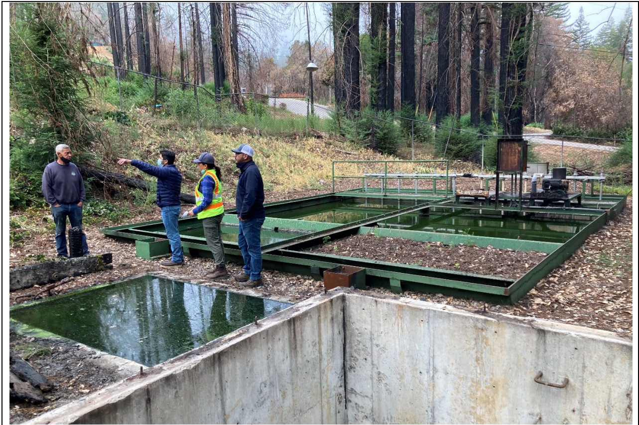
Figure 4: Wastewater basin overflowing. Photos taken by Kent Edler, Assistant Director- Special Services, Santa Cruz County on September 9, 2021
